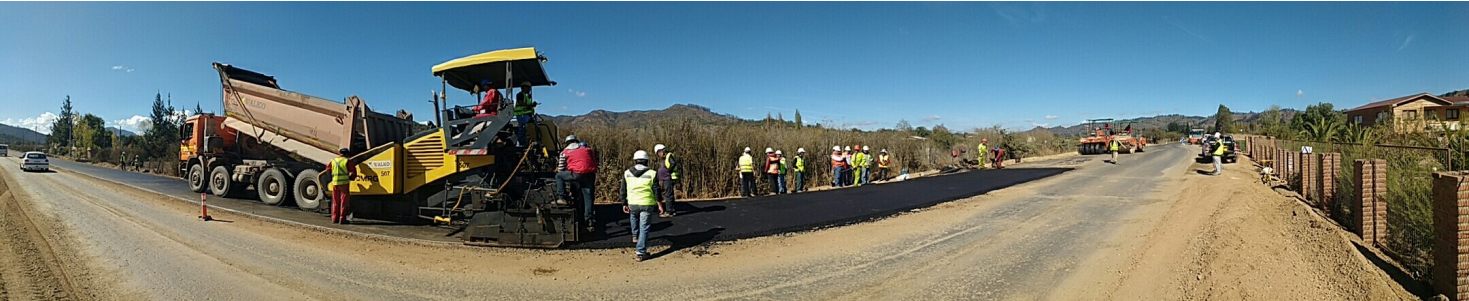
Day 1 on the construction site approximately 100km west of Santiago ... paving and compacting a few hundred metres of black gold
